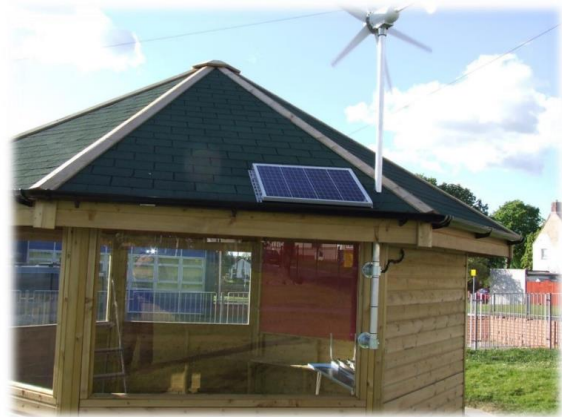
Renewable energy equipment with monitoring board, light and power sockets
