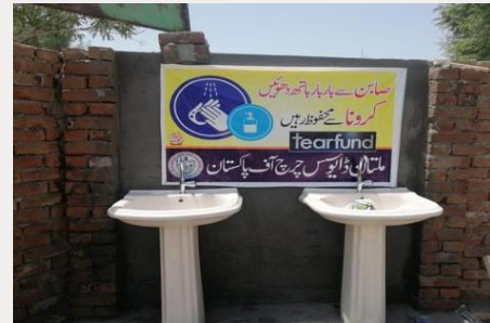
hand washing facilities
