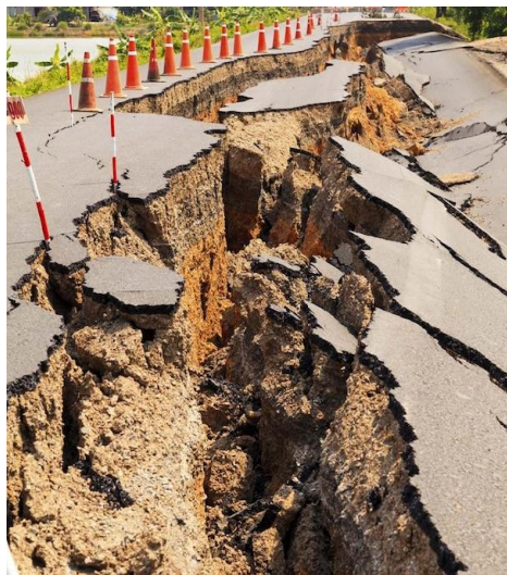
A damaged road which was caused by an earthquake
