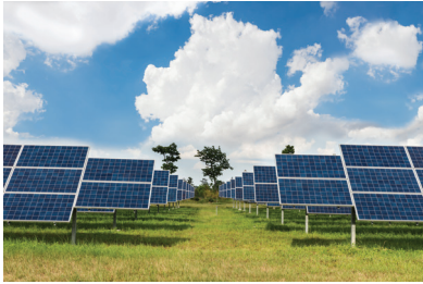
Solar farm in Thailand
